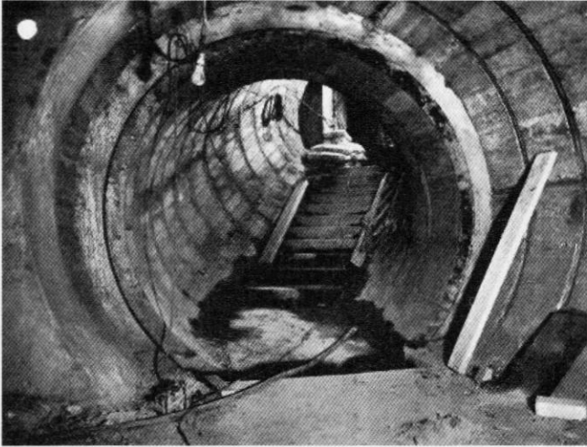
Stairs linking the new lift shaft with the North End station subway during construction of the floodgate control centre in 1956. Photo Colin Tate
